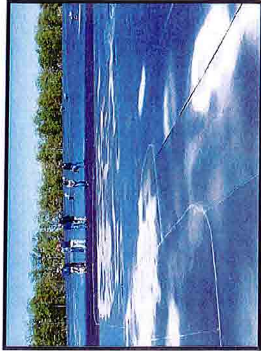
Typical Evidence of Pooling Water on Cap Surface
