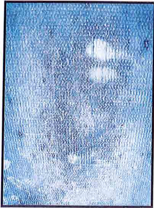
Deterioration on Surface of Liner (typical)
