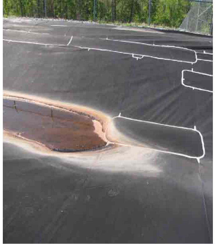
Small area of ponded water on interim cap.
