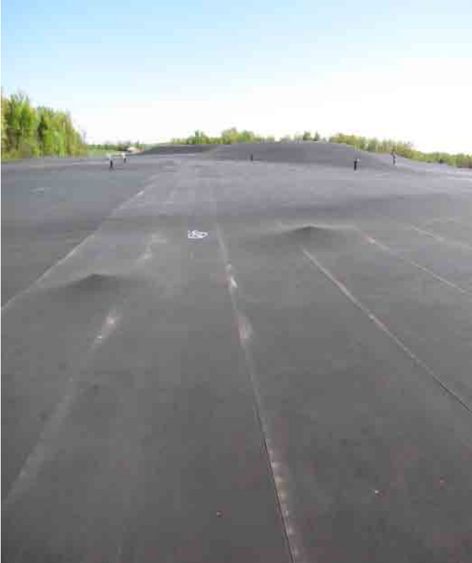
Observed liner "pimples" facing north from southwest portion of interim cap.
