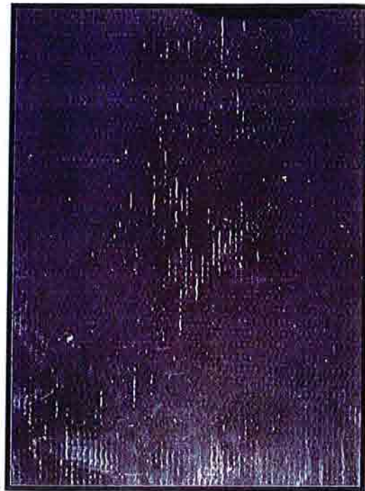
Deterioration on Surface of Liner (typical)
