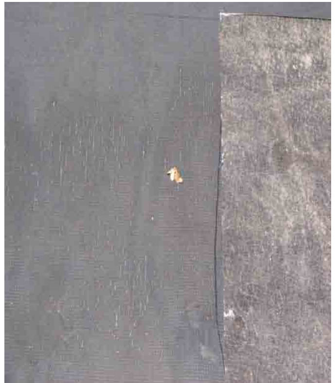
View of liner striations and cut liner sample revealing underlying geotextile.
