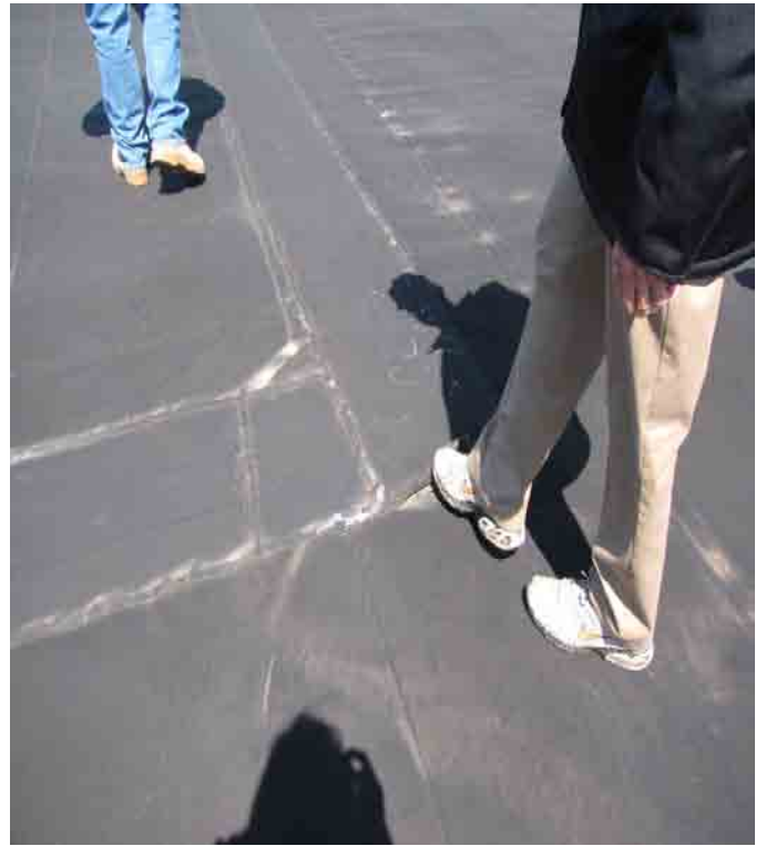
Gap in liner/weld next to the interior diversion berm.
