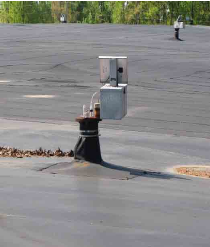
Sump protrusion through interim cap.
