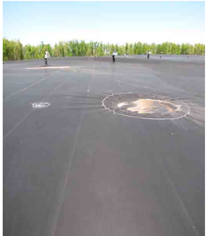
Previous subsidence repair in southeast portion of interim cap.
