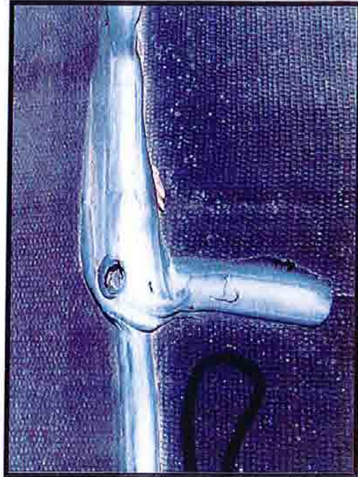
Typical "Bubbling" Failure of Extrusion Weld
