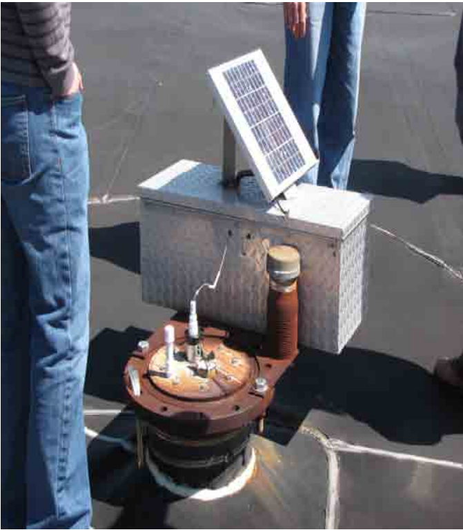
Solar panel for continuous sump level monitors (no longer used).
