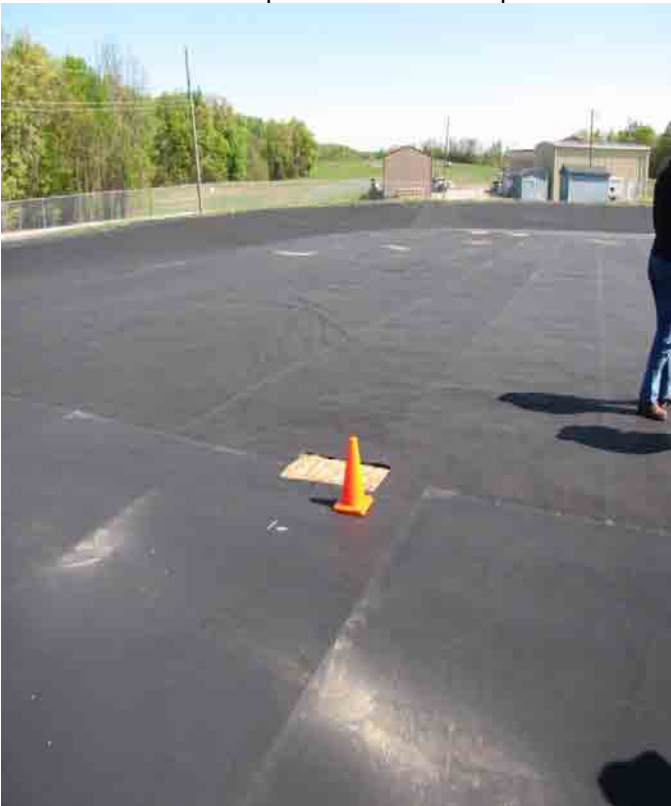
Independent liner inspection liner sample collection in northwest portion of interim cap.
