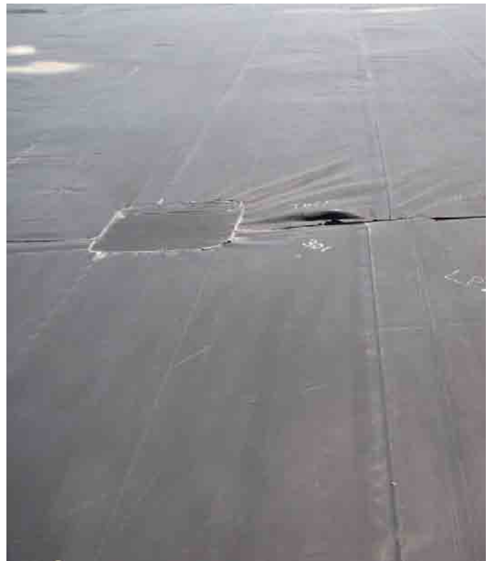
Folded liner material near liner patch.
