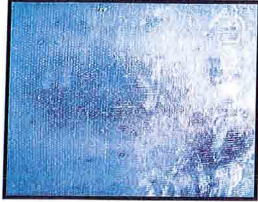
Deterioration on Surface of Liner (typical)
