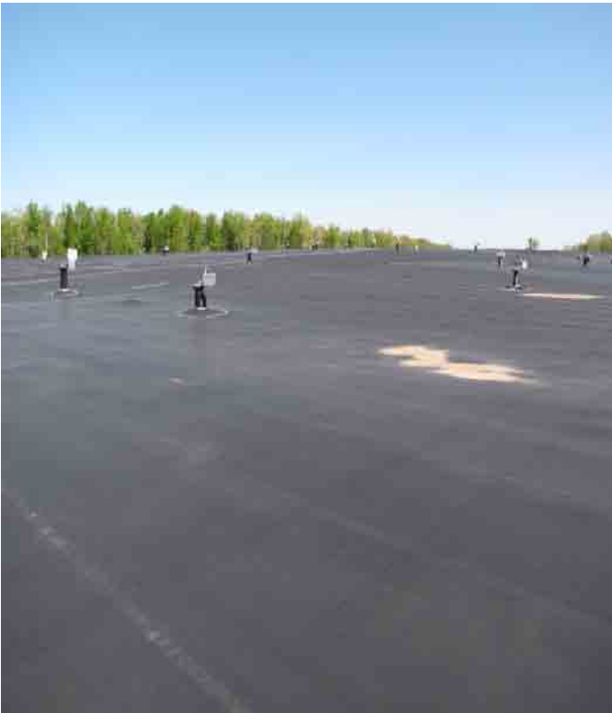
Sump protrusion in interim cap facing northwest from southeast corner.
