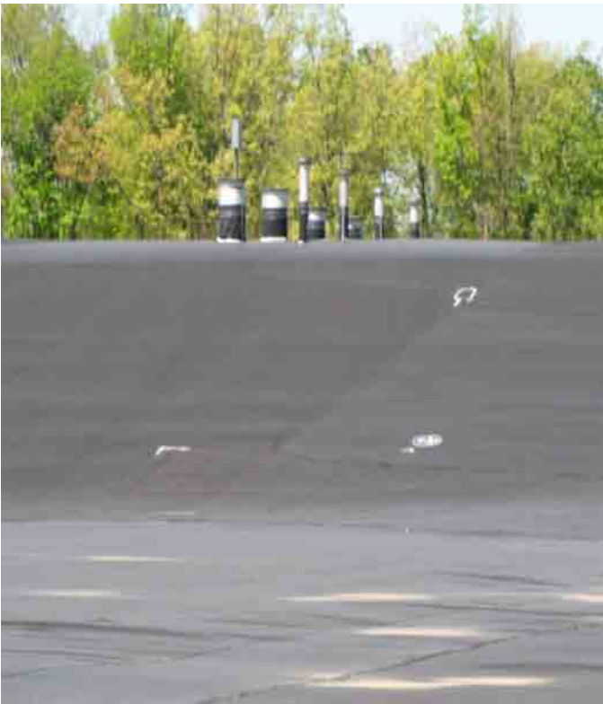
Top of the former leachate storage facility; viewing tank access extensions that are cathodically protected.
