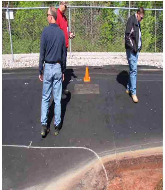
Observed liner striations along SW perimeter of interim cap.
