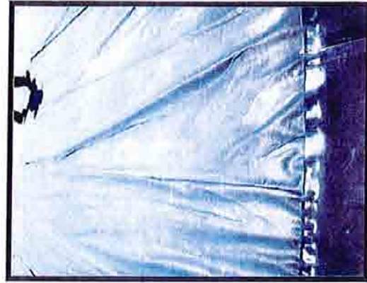
Typical Poor Quality Fusion Weld
