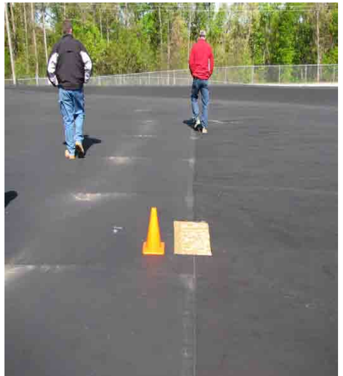
Independent liner inspection liner sample collection in northwest portion of interim cap.
